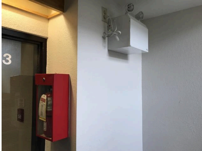
Emergency Lighting Emergency Lighting
