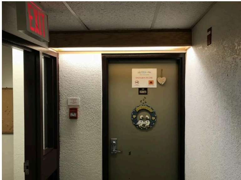
Smoke, Heat Detectors, Fire Alarms Smoke, Heat Detectors, Fire Alarms
