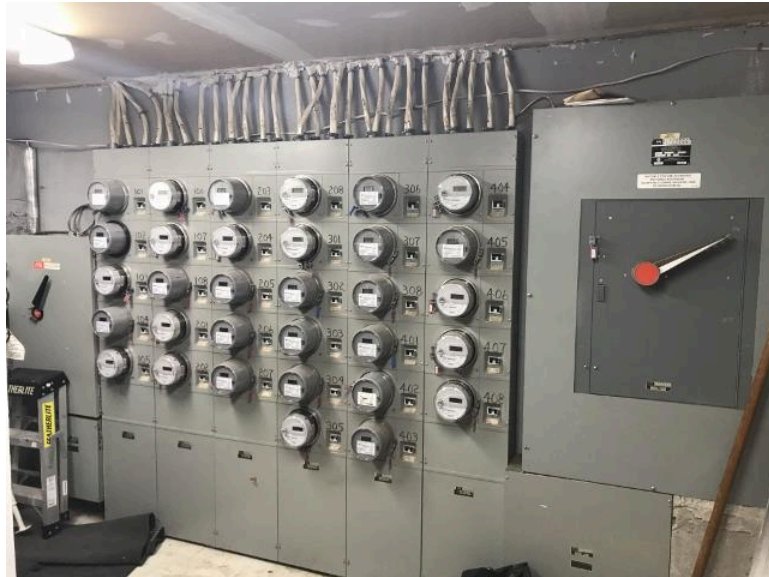
Electrical Supply Electrical Supply
