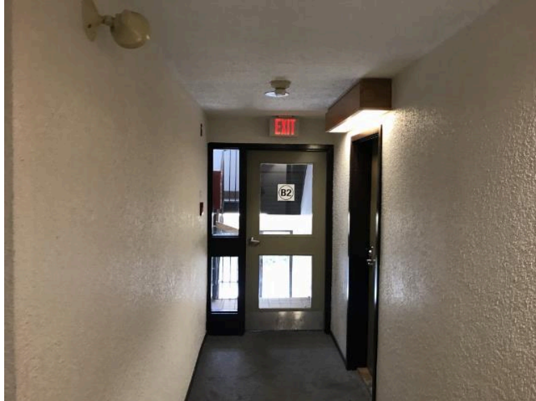
Emergency Lighting Emergency Lighting
