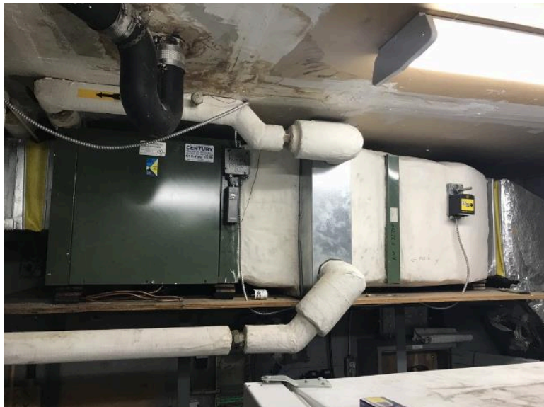
Heating & Ventilation Heating & Ventilation
