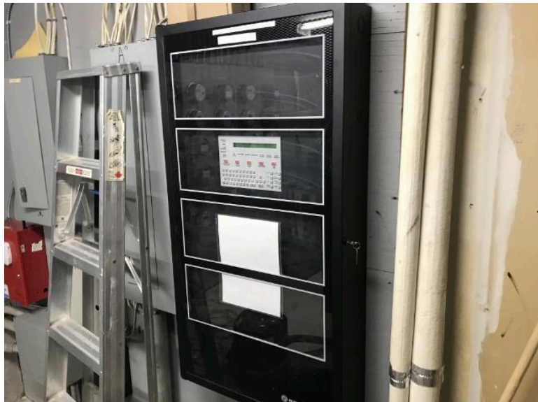
Fire Control Panel Fire Control Panel
